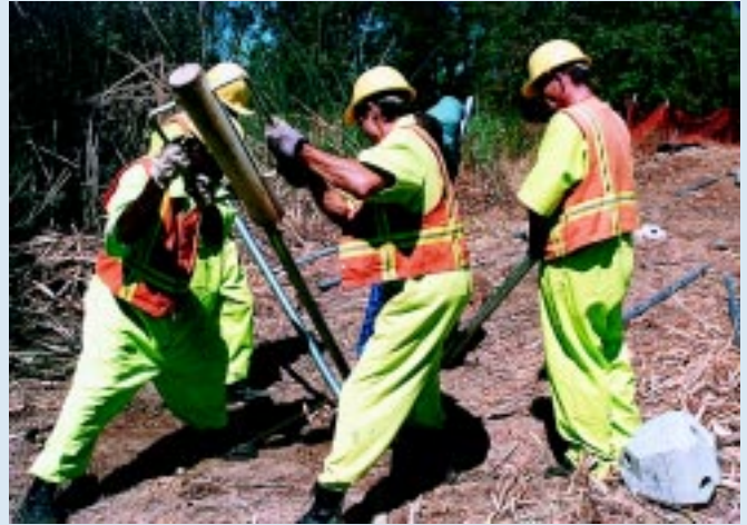
A Folsom Prison crew builds a support for a bridge on the Glenn Drive trail. The men had to use a sledge hammer and jackhammer to complete the task.
